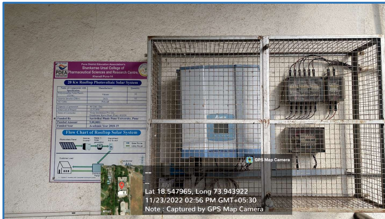
Solar System –Inverter
