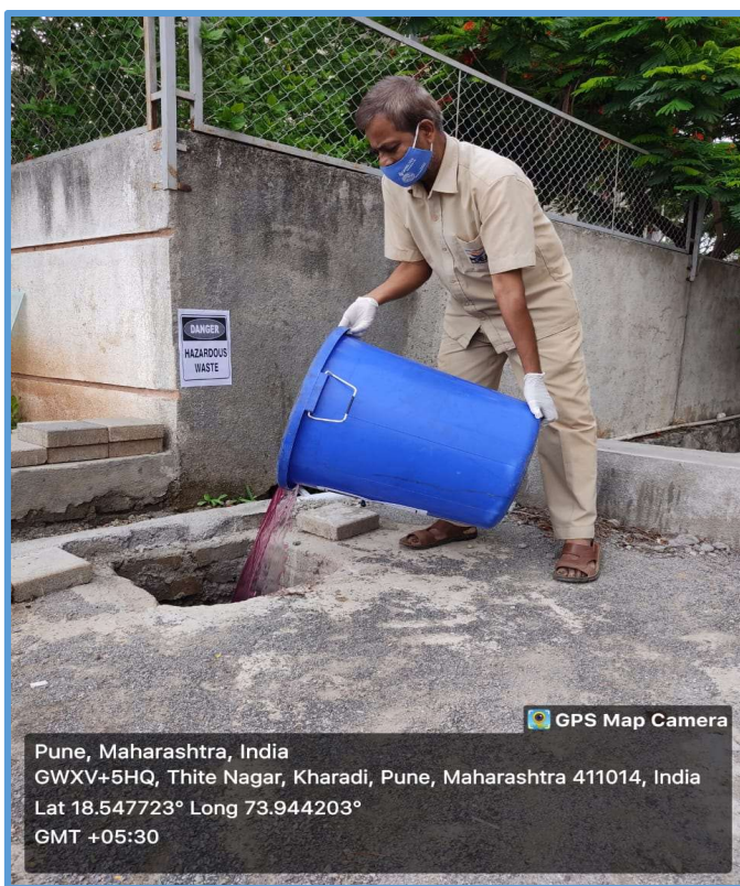
Soak Pit for Hazardous Liquid
