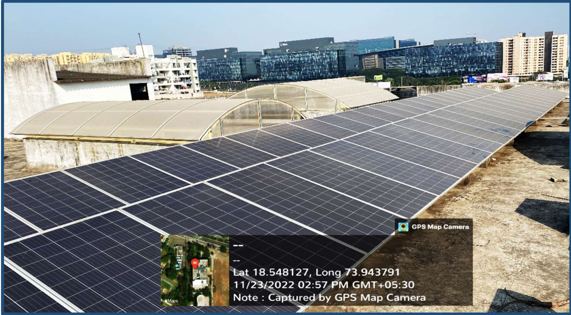
Rooftop Solar Photovoltaic System
